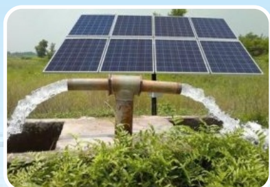
Solar Water Pumping
