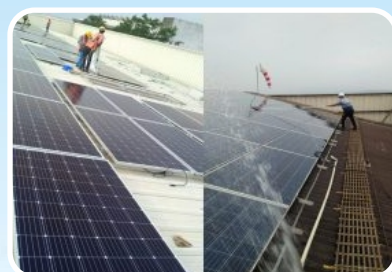
Annual Maintenance Contracts (AMC) / Operation & Maintenance
