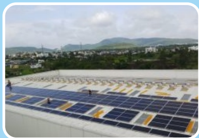
Large Scale PV Power Plant
