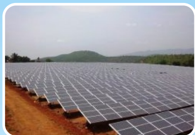
SPV Power Systems:- Ground Mounted, Grid Support & Grid Connected
