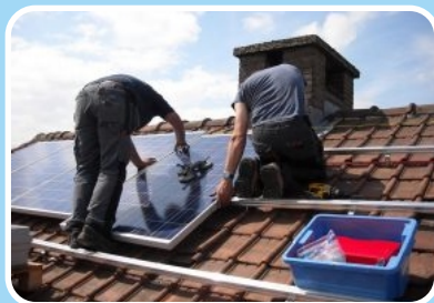
Roofop PV Power Plant
